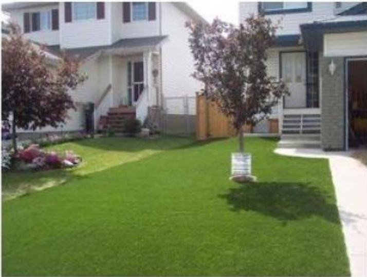
Incorrect – There should be a distinct border installed between the artificial turf and the neighboring natural sod.
